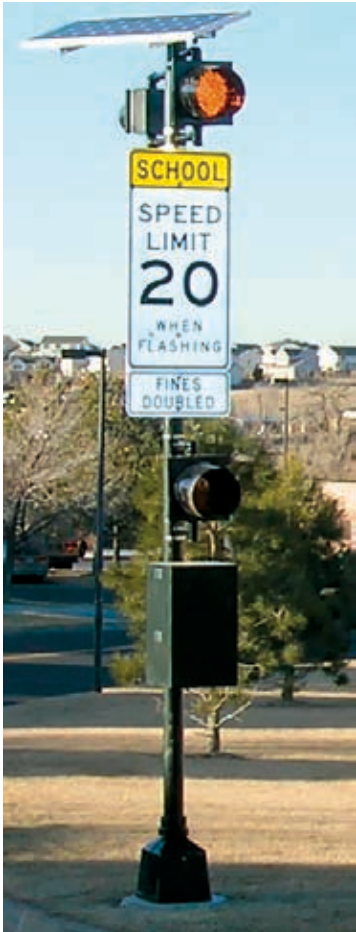
Painted Cabinet and Pole with Confirmation Light
